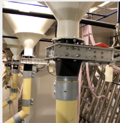
6" (152mm) Roller Gate below hopper handling flour
